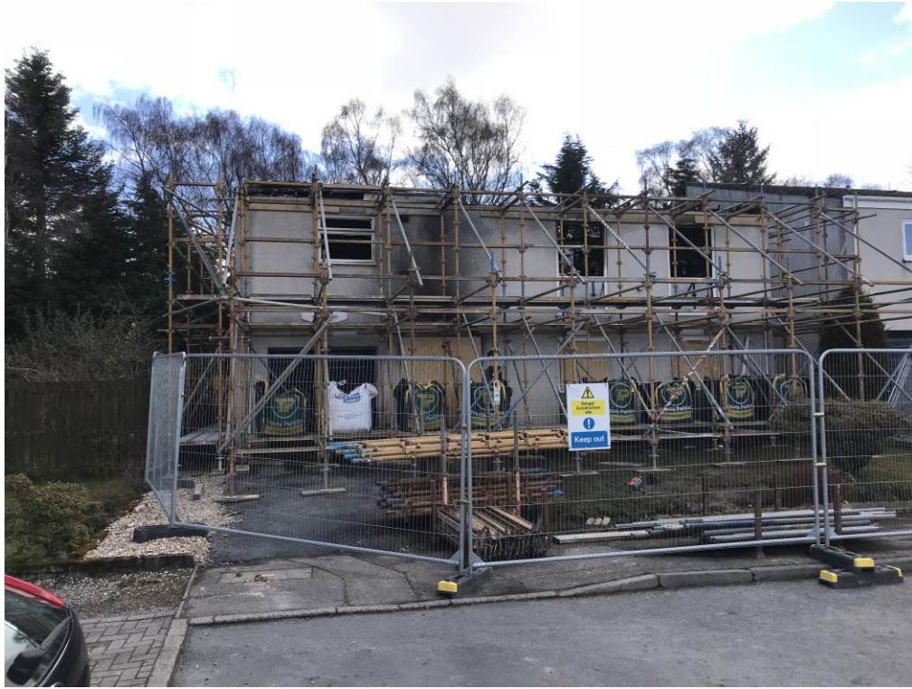
Fire Damaged Property with Support Scaffold Constructed
