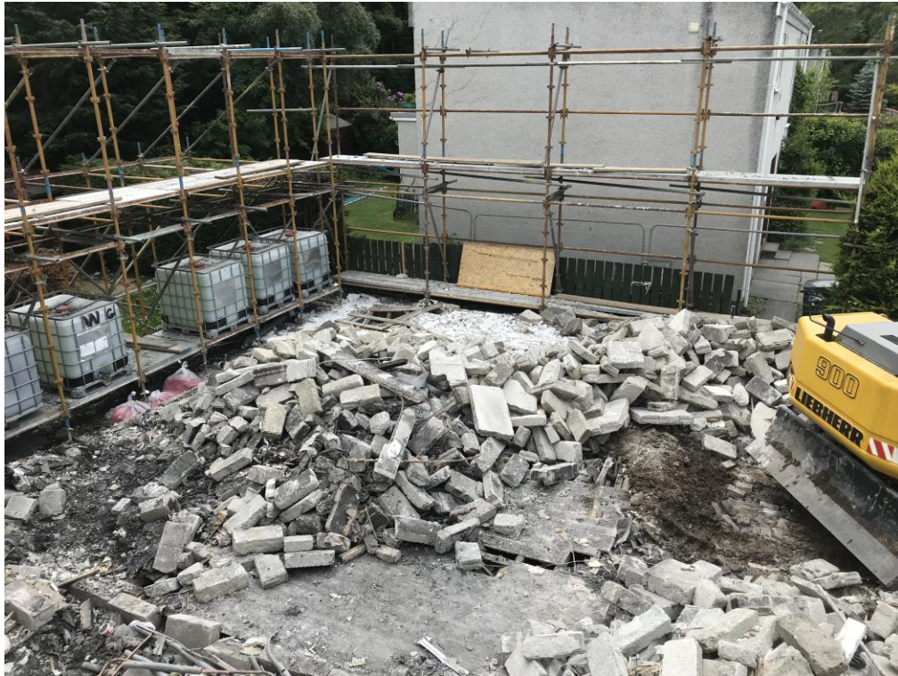
Fire Damaged Property During Demolition
