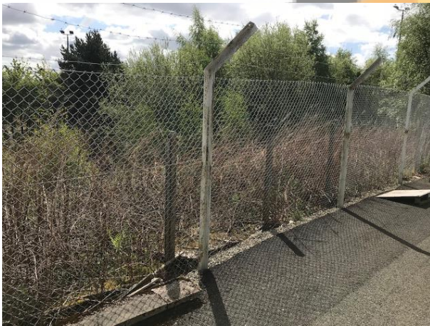
Perimeter Security Fence
