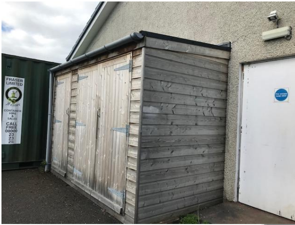
Compressor Store - Locked
