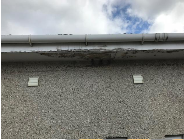
Timber Soffit & Facia – Damaged Paintwork
